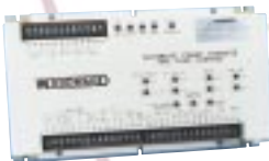
Automatic Power Transfer and Load Control
